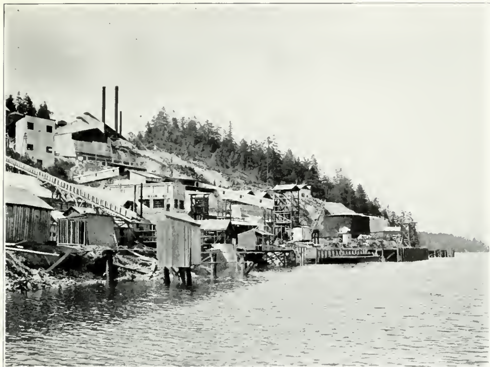
Cement-works, Portland Cement and Construction Co., under Construction at Bamberton, Sunnich Arm.
